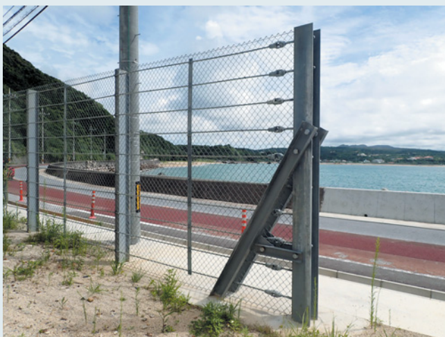
沿岸部の落石防止フェンス支柱 Steel posts of guard fence at coastal area
